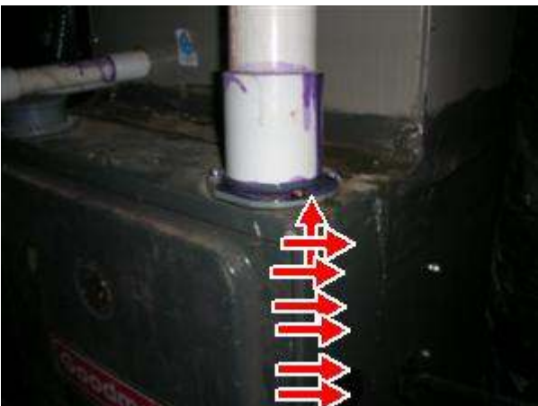
A. Picture 1 water running down furnace
